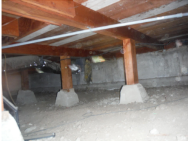
Area under uneven floor at right-front of original structure
