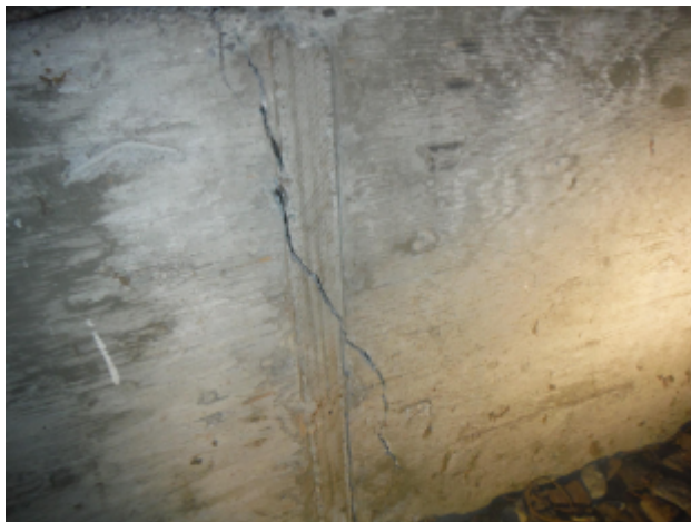
One of three vertical cracks in the foundation
