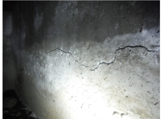
One of two horizontal cracks in the original foundation
