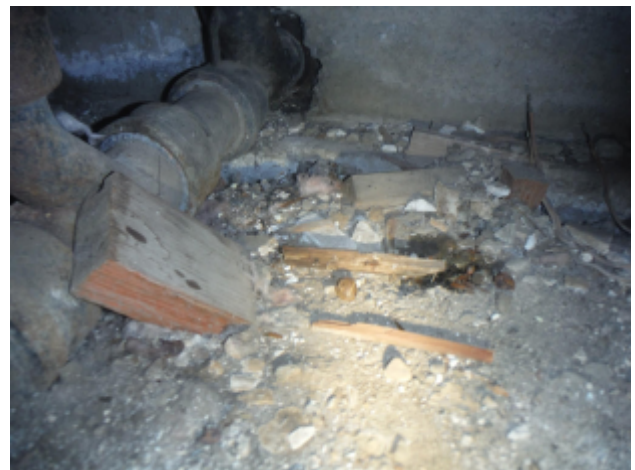
Example of cellulose debris in the crawl space
