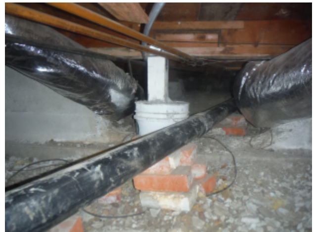
Restricted clearance at access to right-rear addition
