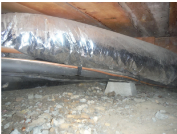
Restricted clearance under right-rear addition
