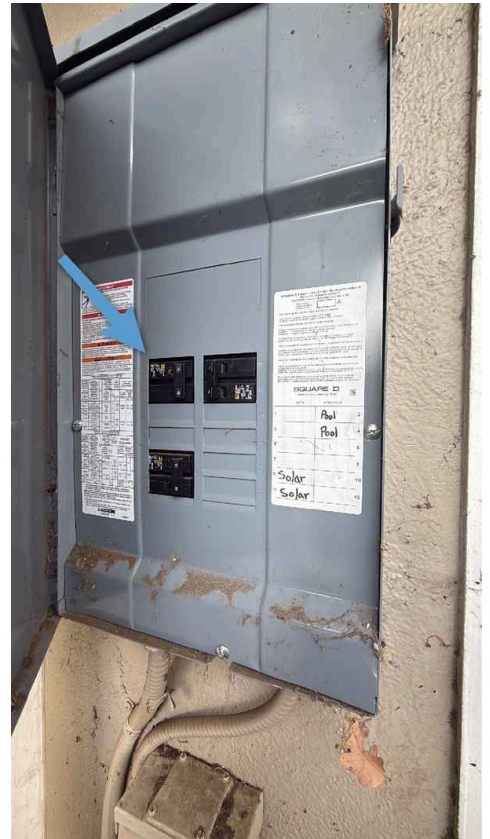
Exterior sub panel
